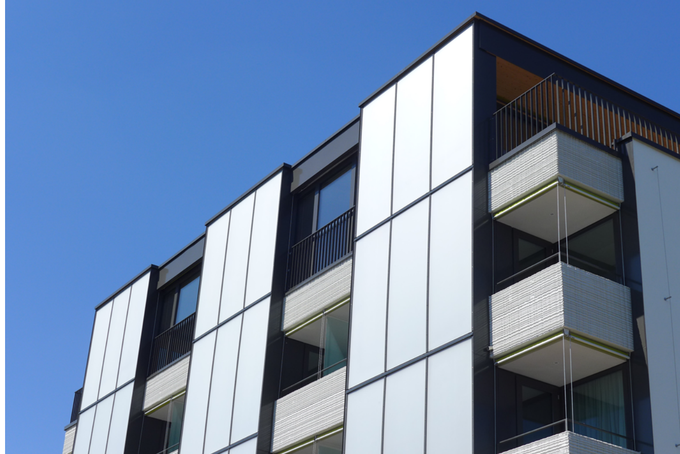
Solar thermal façade collectors on apartment building, Switzerland
