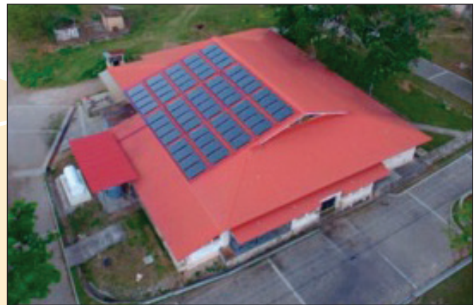
▲ Figure 4. Solar thermal system at a dairy plant in Honduras. (Source: SOPELIA)
