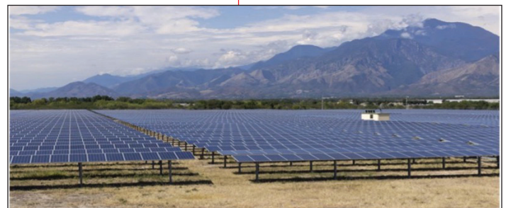
▲ Figure 3. SIBO Solar Power Plant in Guatemala. (Source: MEM, Guatemala)
