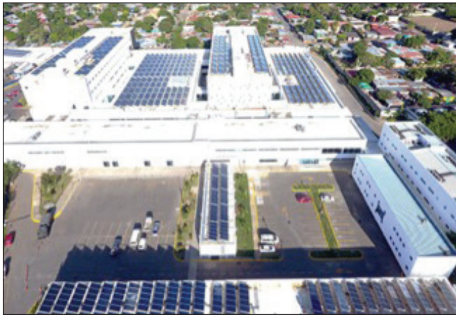
▲ Figure 5. Solar thermal installation on a Nicaraguan hospital. (Source: Hospital Militar Escuela Dr. Alejandro Dávila Bolaños)
