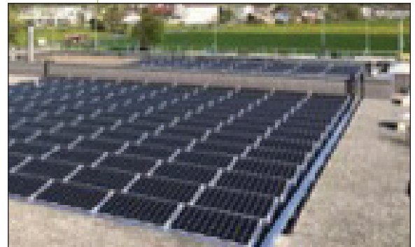
▲ Figure 3. In Switzerland, this PVT system uses 178 uncovered PVT panels + 699 PV modules to generate 237 kWp. The heat pre-heats the groundwater storage, which is then transferred directly to the heat pump and the overflow basins of the pools. The heat pump generates heat for pools, space heating, and domestic hot water. A gas boiler supports the heat pump for peak loads. Electricity is for self-consumption and the grid. (Credit: Meyer Burger)
