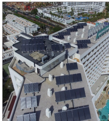
◀ In Spain, the conditions are suitable for a low payback time. 102 PVT glazed panels covering 200 m 2 generate 30 kWp to provide hot water and electricity for self-consumption and the grid at this hotel. (Credit: Abora Solar)
