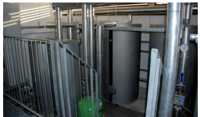
↑ Illustration 250 : Insulation of the distribution network
