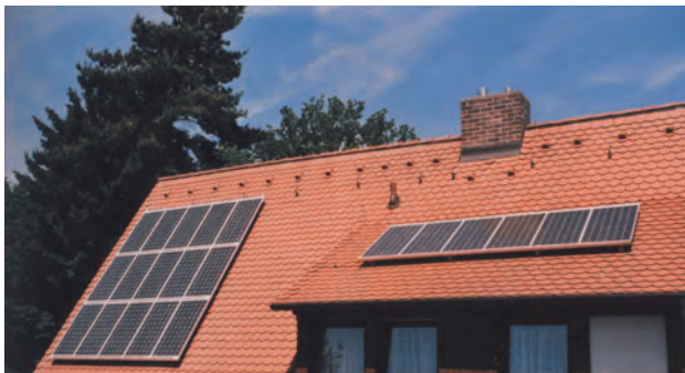
↑ Illustration 316 : The solar collectors, with different orientation, must be connected in parallel
