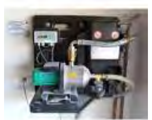
↑ Illustration 353 : Pump installation
