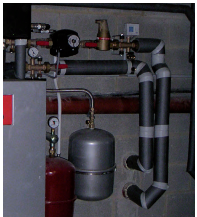
↑ Illustration 233 : Insulation of the distribution network.
