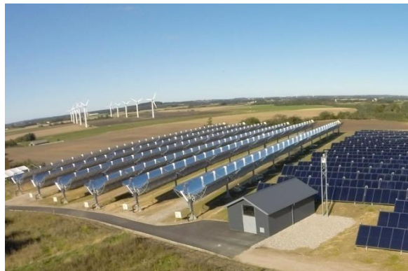
Figure 6: Combination of flat plate collectors and parabolic trough collectors in Taars, Denmark (Aalborg CSP)
