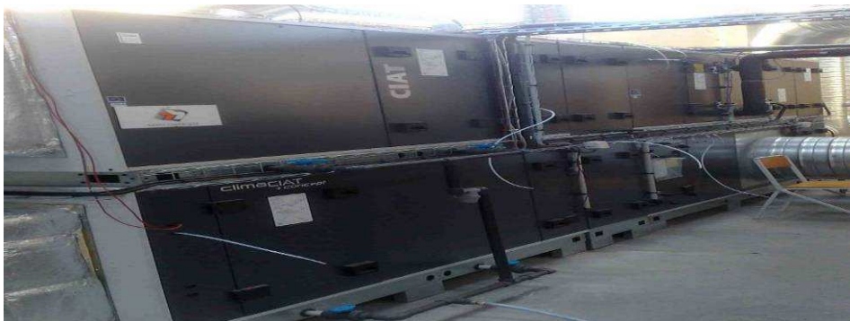
Figure 6: Experimental solar desiccant cooling installation of La Rochelle
