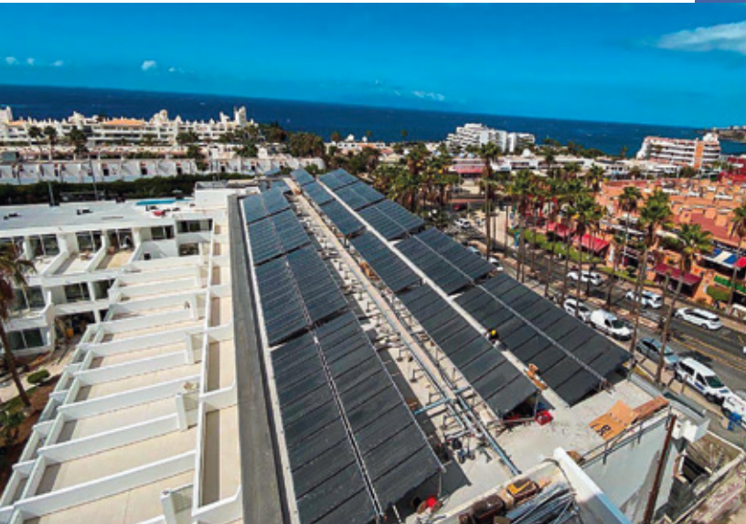
Photo: Abora Solar, Spain
