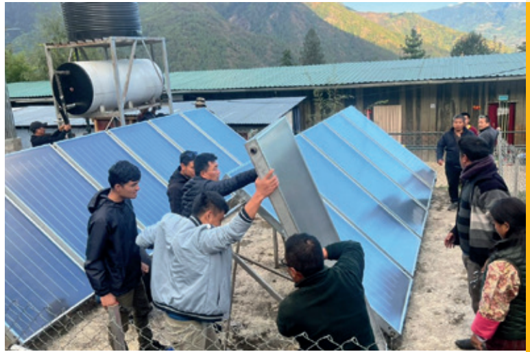
Installation of a ground-mounted solar thermal hot water system in Bhutan
