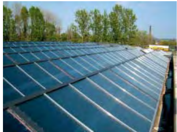
Solar plant 'AEVG Graz' (currently 3,550 m 2 , total ~5,000 m 2 ) for feed-in into district heating net, employing Gluatmugl HT collectors. Engineering by S.O.L.I.D. GmbH
