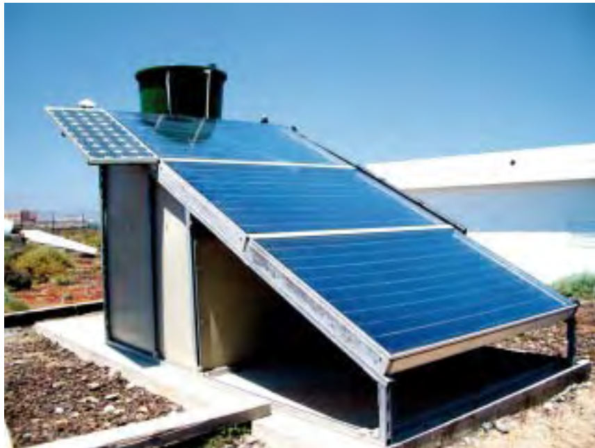
Double-glazed AR collector from ESE used in a solar driven desalination system installed December 2004 in Gran Canaria, Spain. The collectors and the desalination system are still in operation and have shown very good performance.
