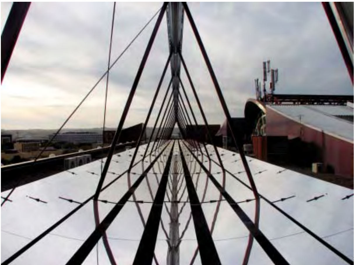
The PSE linear Fresnel Collector in Sevilla, Spain
