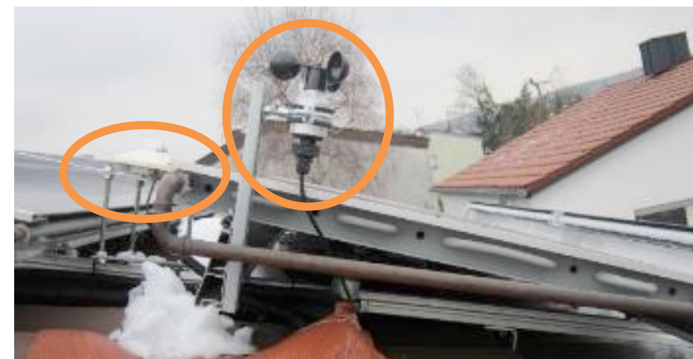
Monitoring equipment, IGTE
